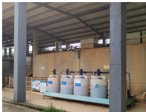
污水站加药区
