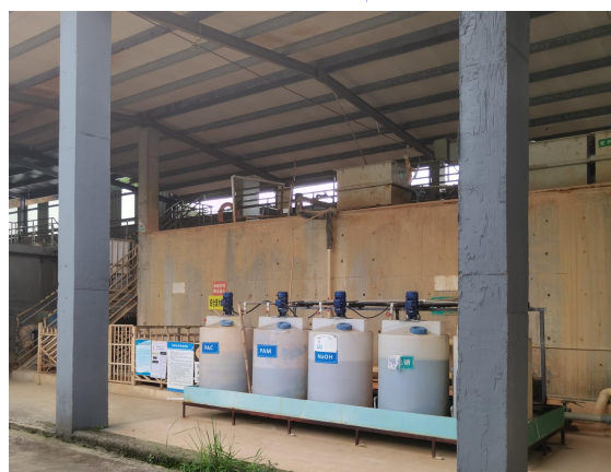
污水站加药区
